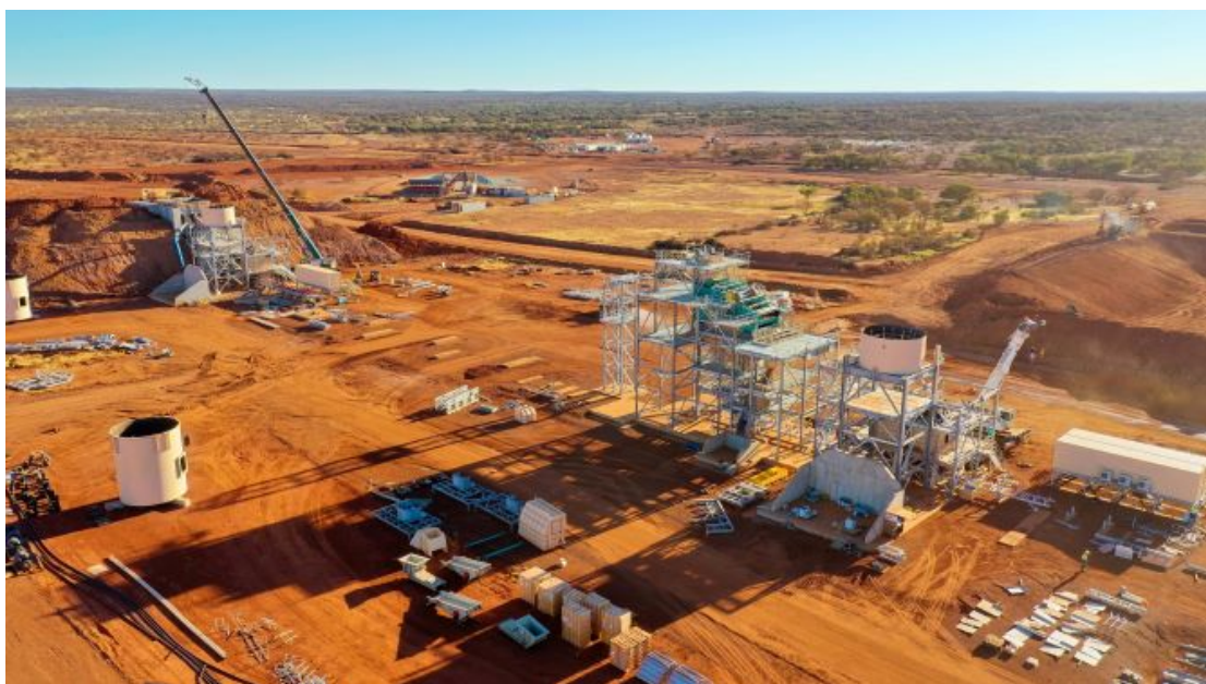
Primary, secondary and tertiary crusher installation
