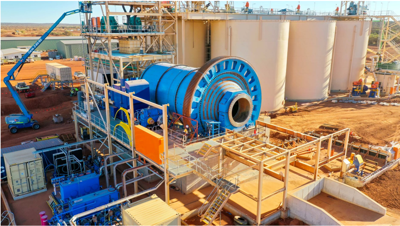
Mill and CIL tank area
