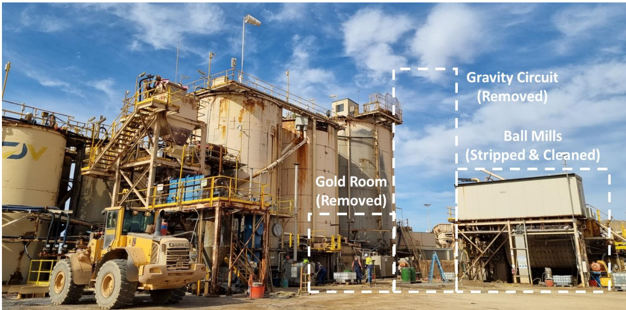
Fig 4 – Central Gawler Mill with gravity circuit, gold room and other key equipment removed 11
