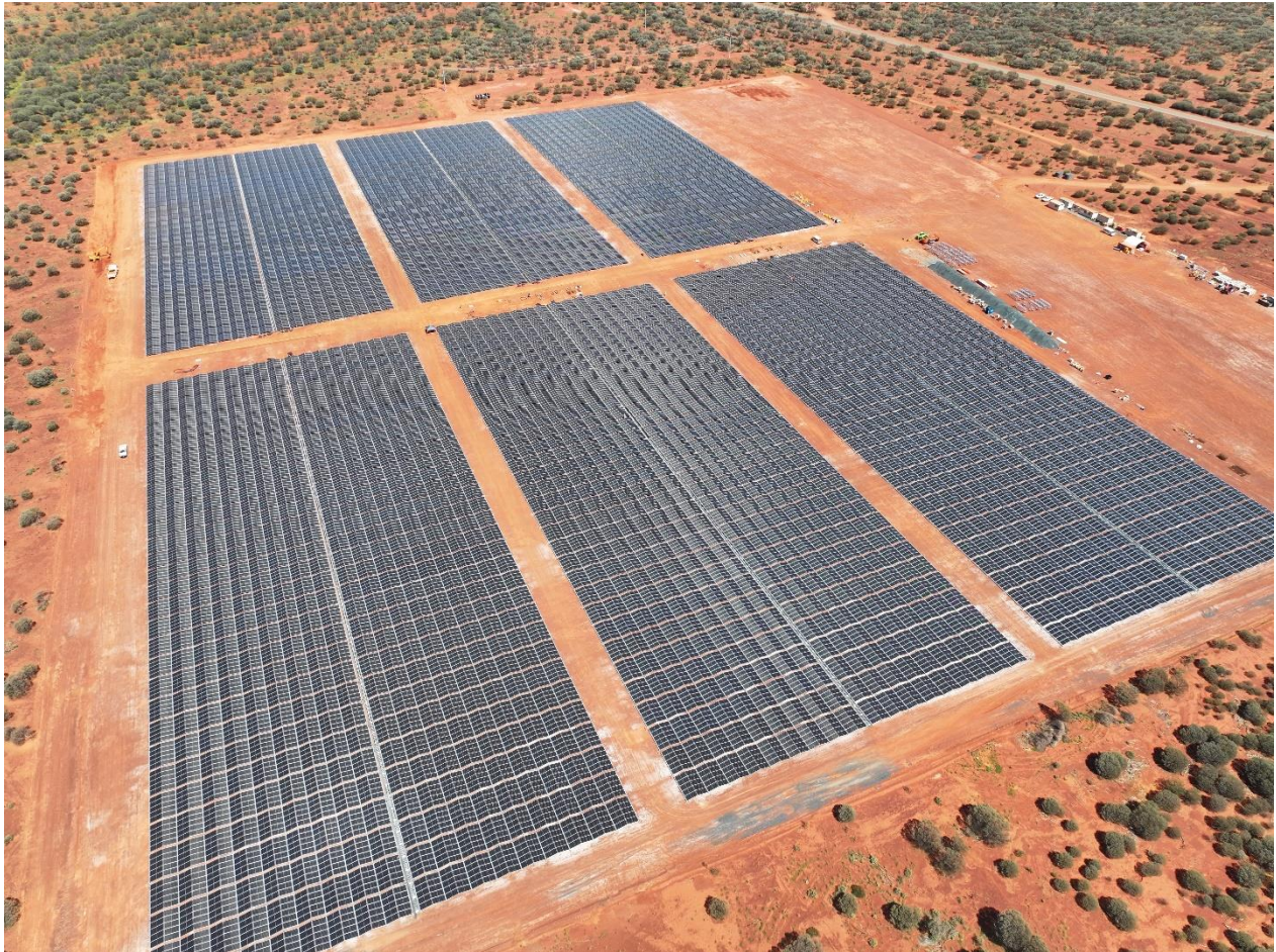
Figure 8: Installation of first 20MW of renewable energy solar power, progress as at 6 April 2024.
