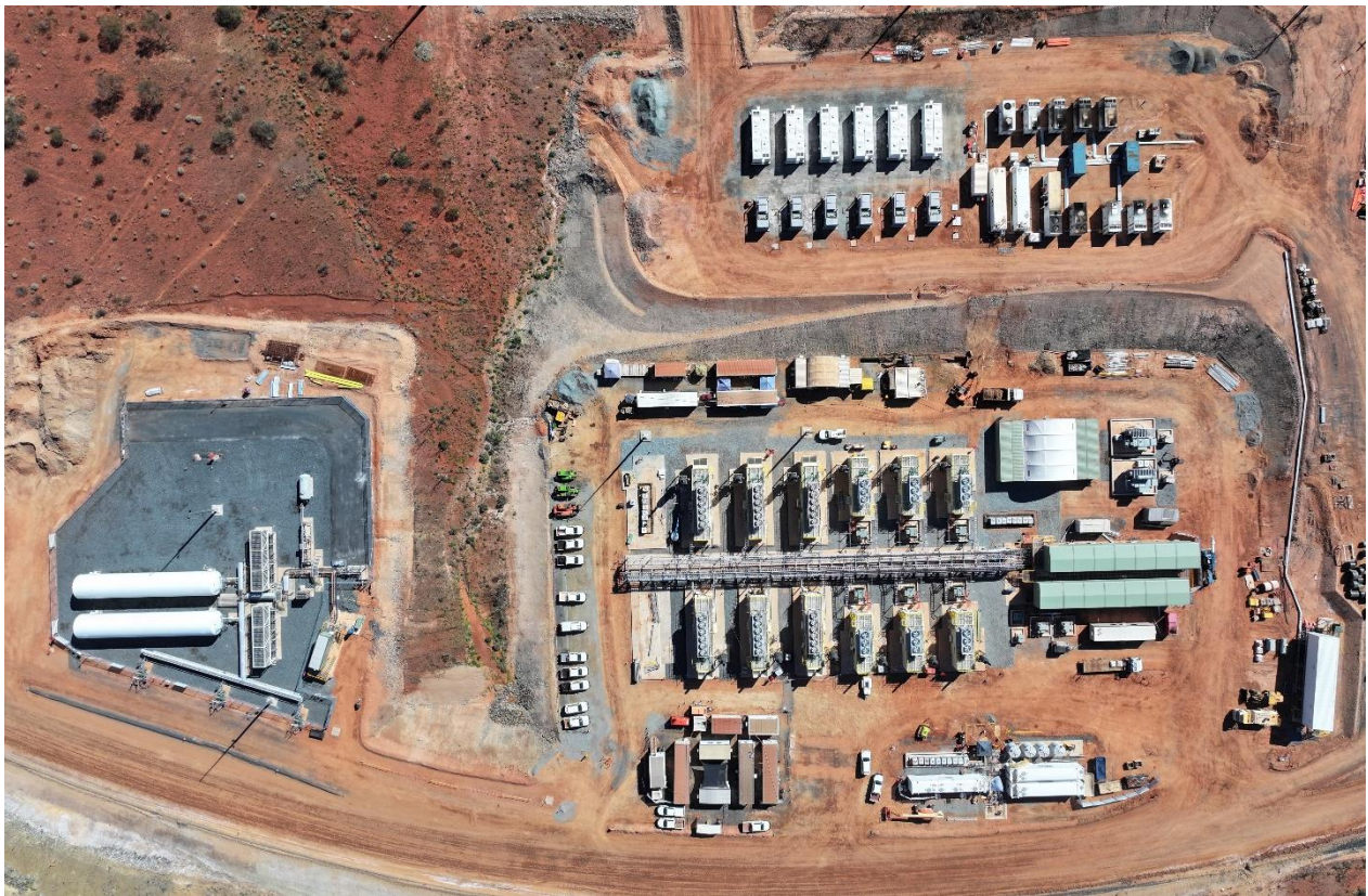
Figure 7: Thermal power station progress as at 9 April 2024 – construction complete and commissioning underway.
