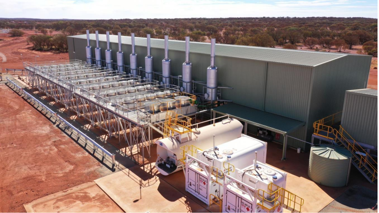
18MW power station operational
