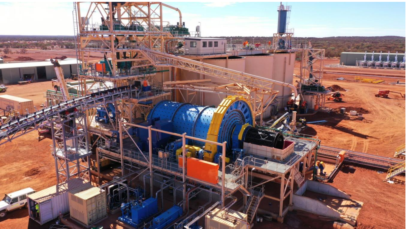
7.5MW ball mill installed aligned and fully rubber lined. VSD motor commissioning underway.
