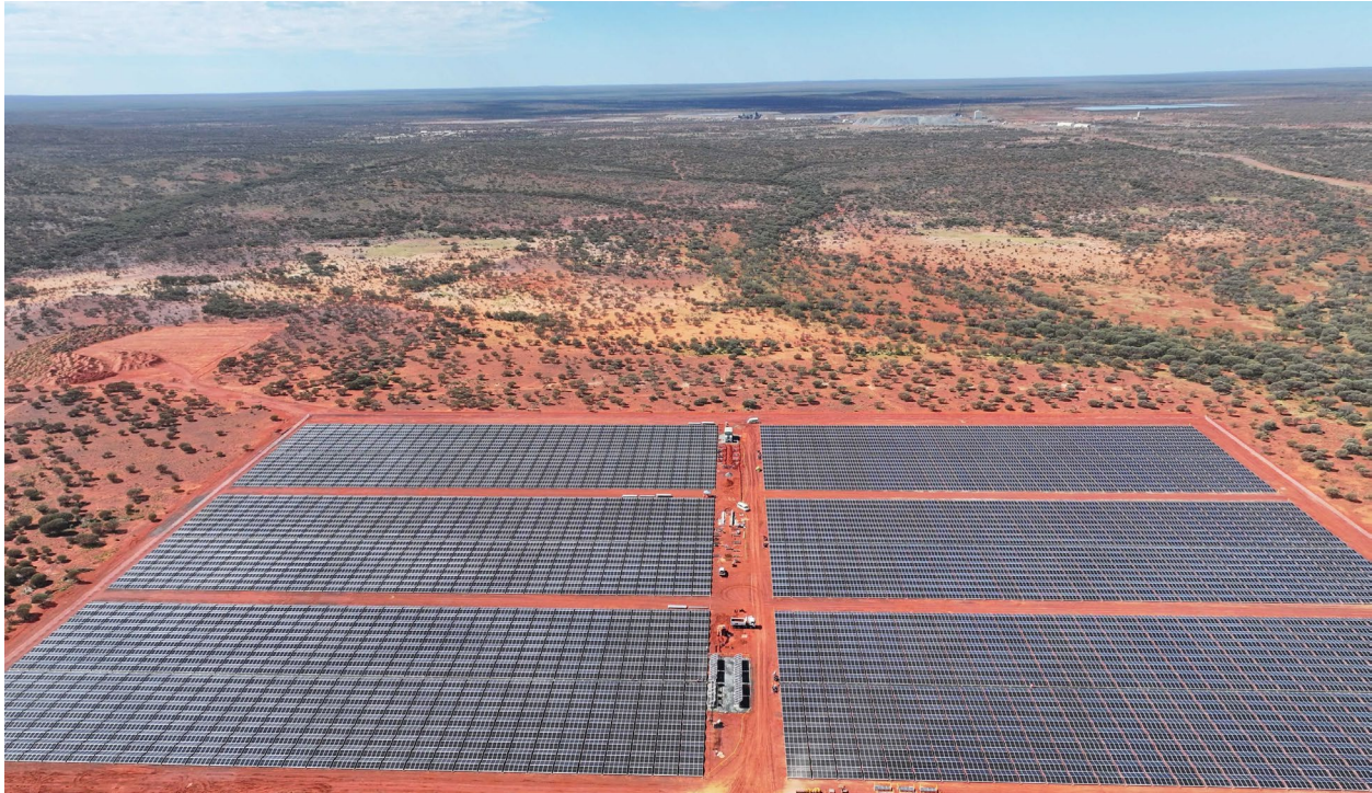
Figure 1: 20MW Solar Array at the Bellevue Gold Project.
