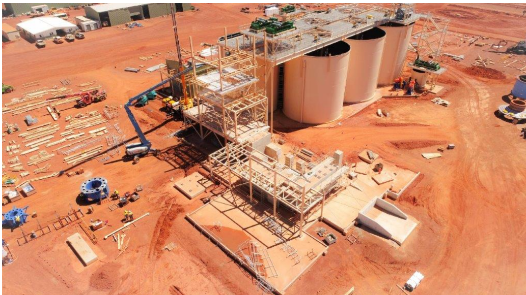
Mill and CIL tank area
