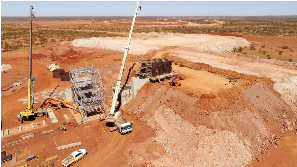
Primary and secondary crusher area
