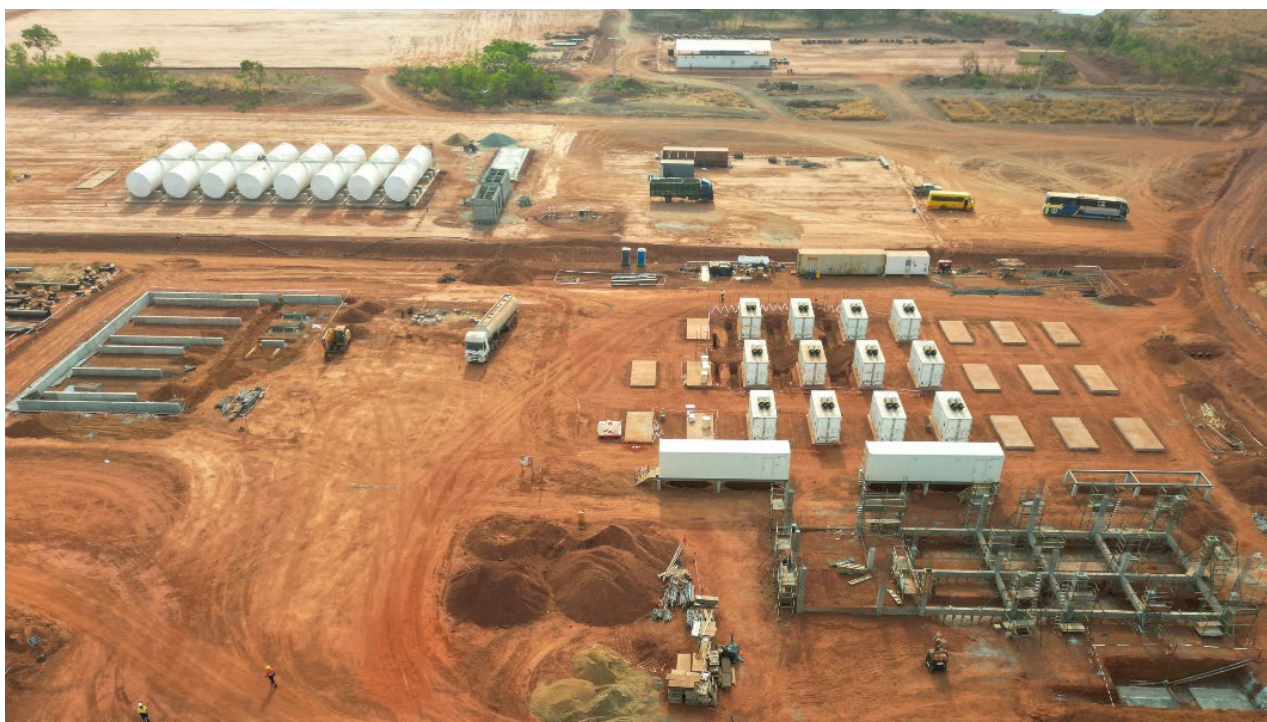
Image 10: Power plant and fuel farm
