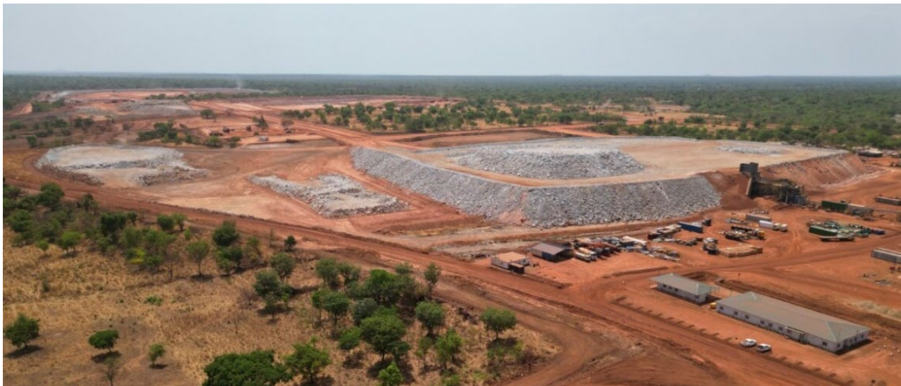
Image 4: ROM pad construction complete and ore stockpiling has commenced on the first ROM finger.
