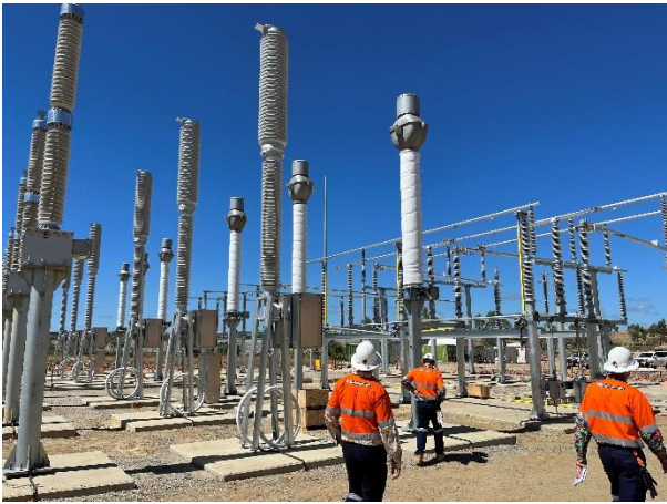
Figure 3: K2H Switching Station
