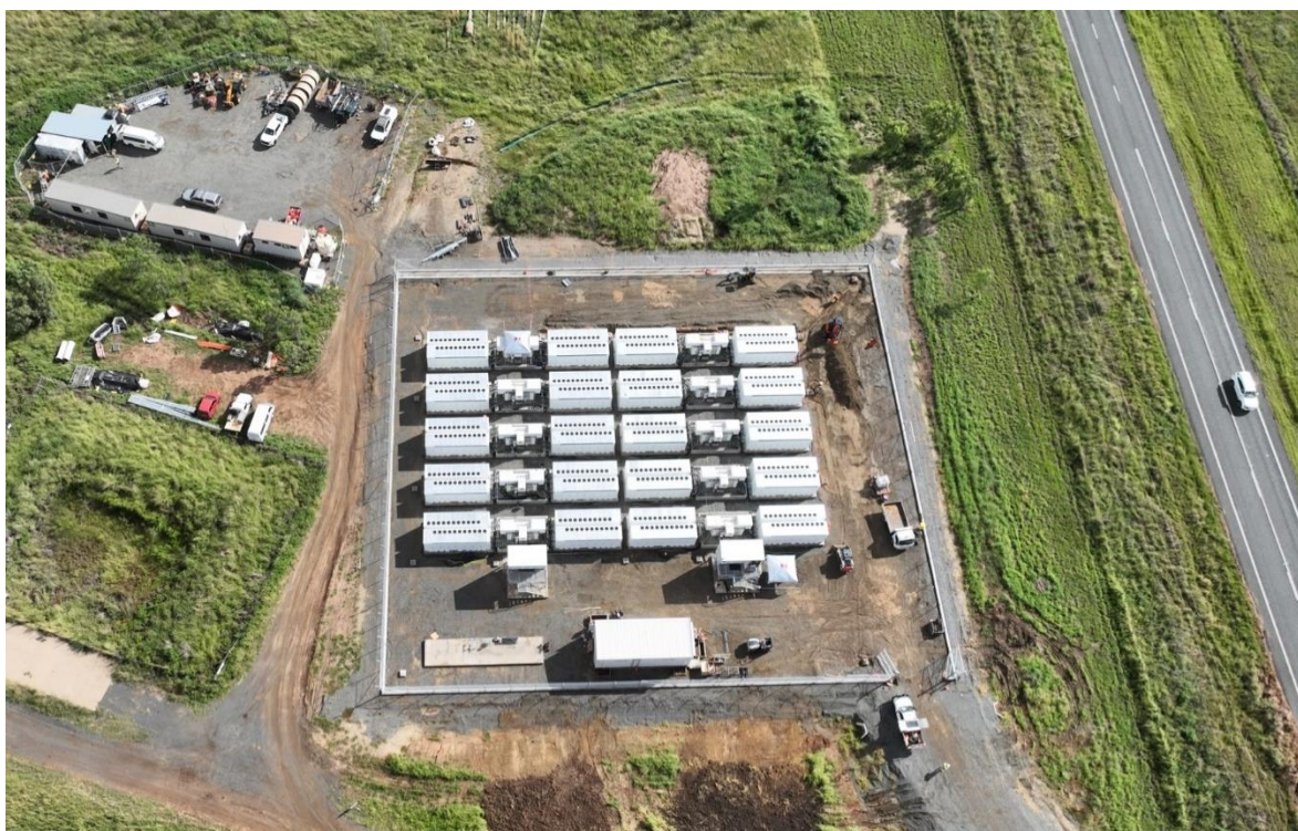
Figure 7: 50MW/100MWh Bouldercombe Battery Project
